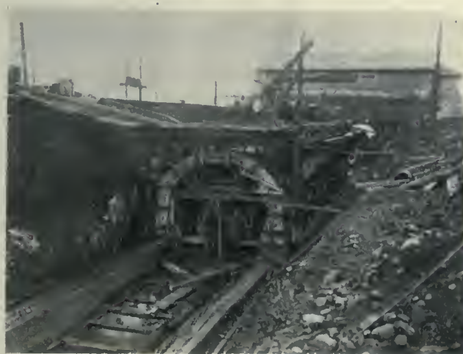
First completed section of aqueduct—Buggies used for conveying concrete from the mixers on pouring platform—Forebay in background.
